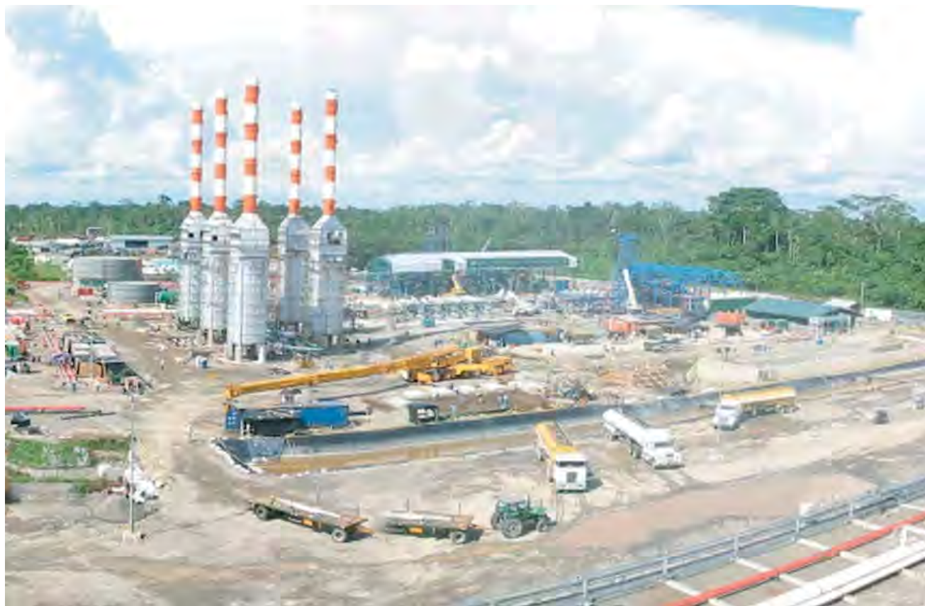
OCP, Amazonas (Ecuador) - n° 5 Hot Oil Heaters.
