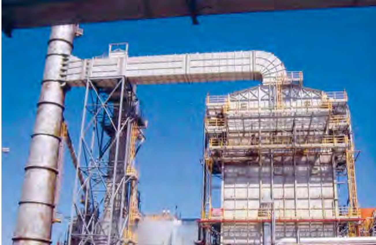
PETROCHEMIA , Plock (Poland) UOP Product Fractionator Feed Heater.
