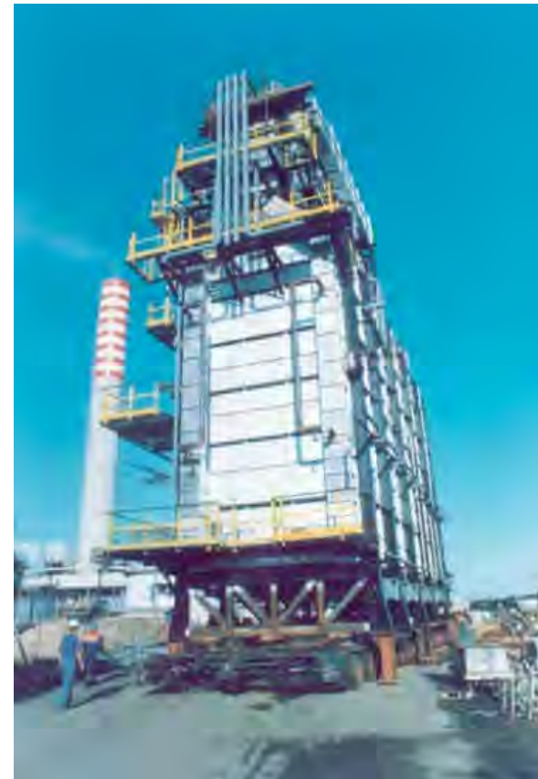
Shifting of the new heater (450 tons) in one piece, using same trailers.
