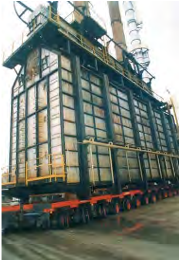
Shifting of the old heater (450 tons) in one piece, using self-propelled platform trailers.
