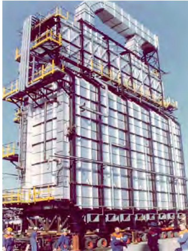
Shifting of the new heater (450 tons) in one piece, using self-propelled platform trailers.
