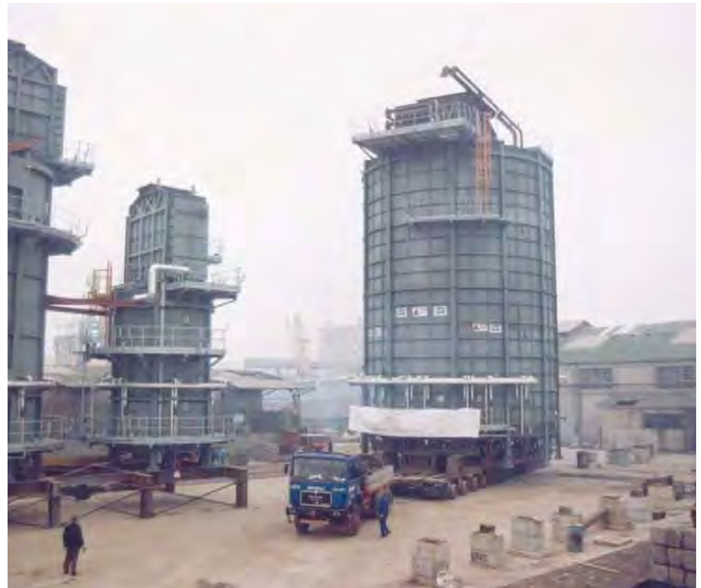
Hydrofiner & Hot Oil Heater
